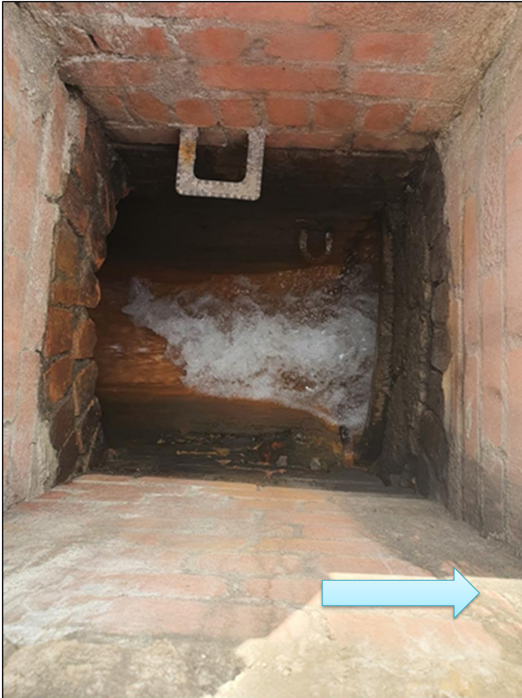
Photograph 4 View of inside inspection chamber that was blocked during Storm Dennis. Arrow shows direction of flow of water. Water is flowing freely and unobstructed. (June 2021)
