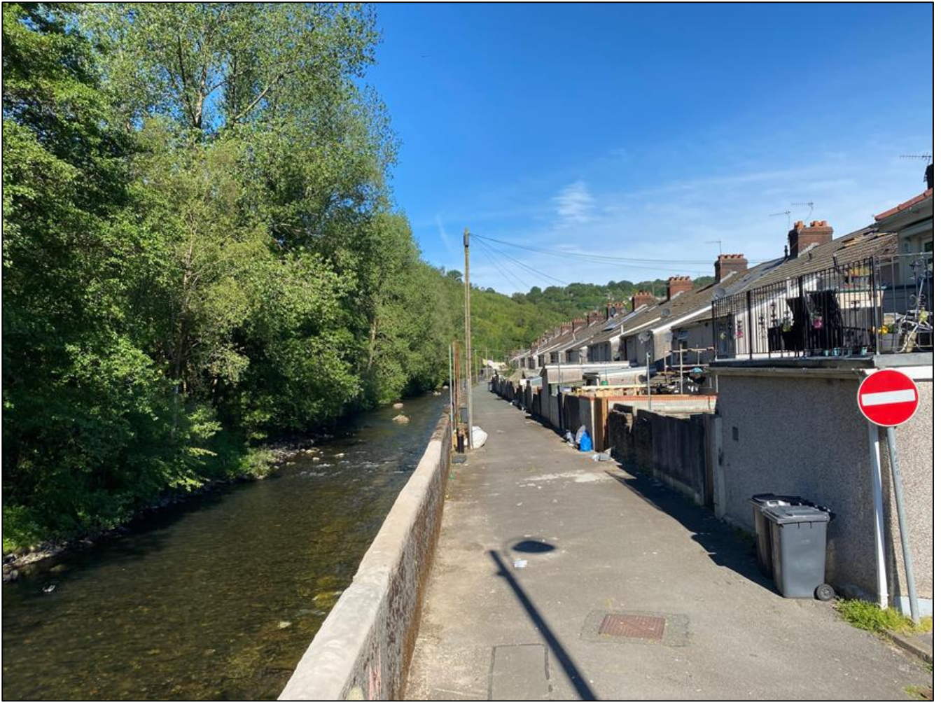
Photograph 8 Rear of Meadow Street along the bank of the River Ebbw. NRW's flood defence wall protected the street from fluvial flooding. View West. (June 2021).
