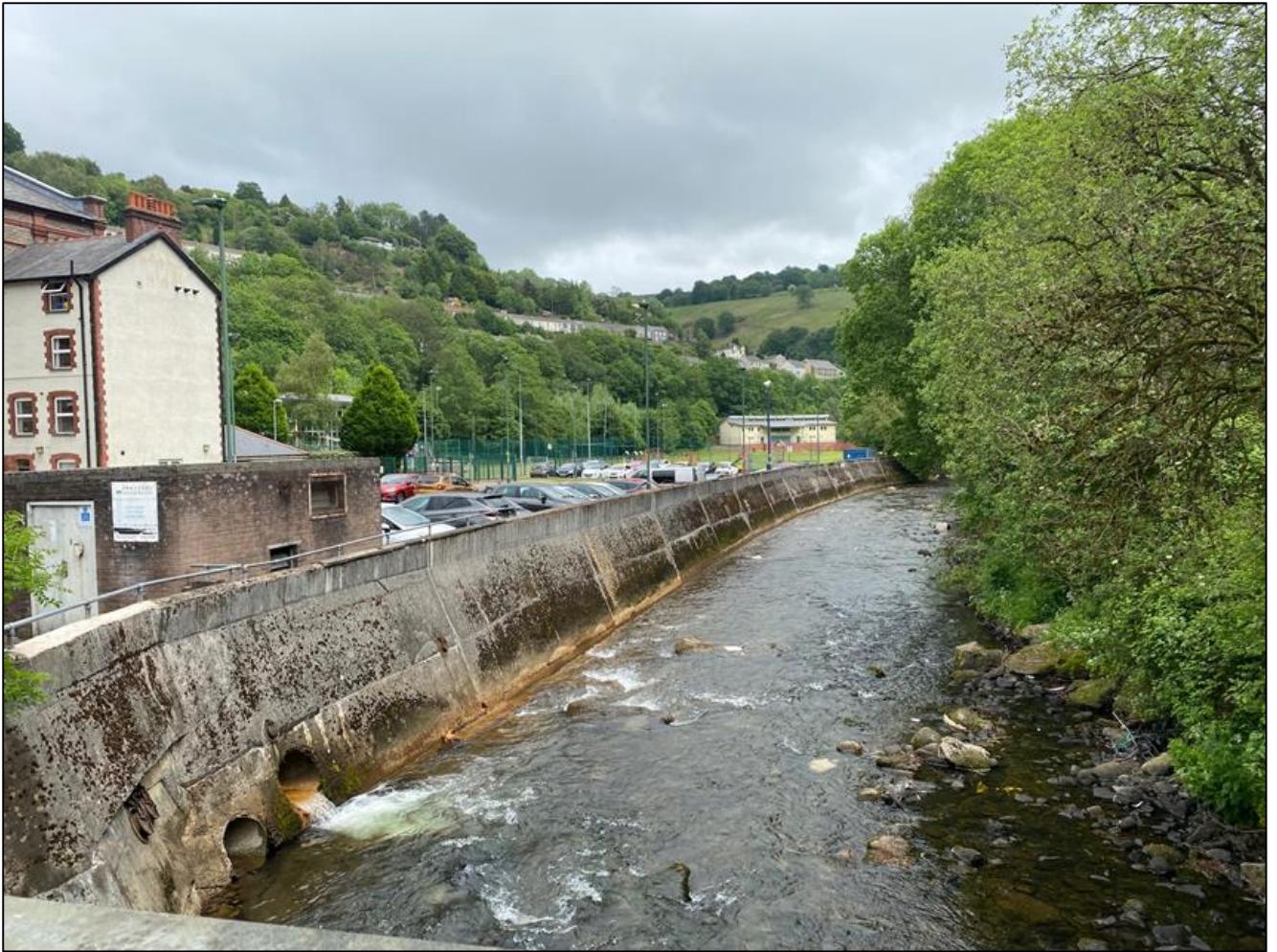
Photograph 9 The River Ebbw flowing in a south easterly direction. At the bottom lh side of the picture is the outfall of the Nant Cuffin Culvert and pumping station inlet. Above the outlet is DCWW's pumping Station building. In the distance is the car park for St Illtyd's Primary School and Llanhilleth's Recreation Ground. (June 2021).
