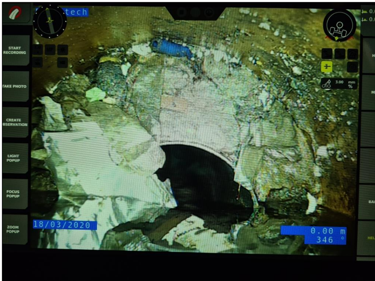
Figure 5 CCTV Survey footage of the outlet pipe covered with debris
